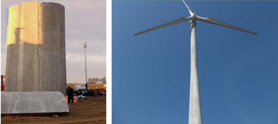
Figure 1.14. Rounded square base of Potensa Wind Tower (left) (Potensa Wind Structures, 2016); taper from square to circular section in completed tower (right) (Ericksen Roed & Associates, 2015)
